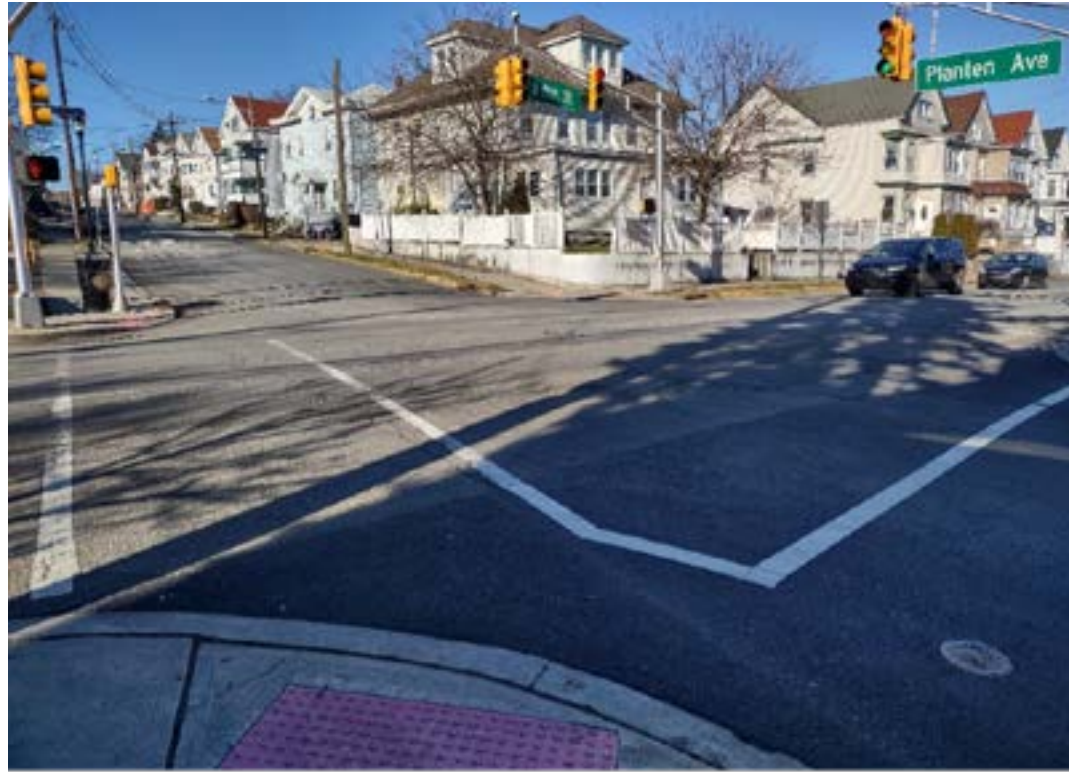
FIGURE 8 FROM THE SOUTHWEST CORNER OF THE INTERSECTION, LOOKING NORTH, ARE FADED AND BARELY VISIBLE MARKED CROSSWALKS AND TRAVEL LANES. ADA WARNING PADS ARE PRESENT, BUT ARE NOT POSITIONED CORRECTLY IN ORDER TO PROVIDE PHYSICAL CUES TO BLIND INDIVIDUALS.
