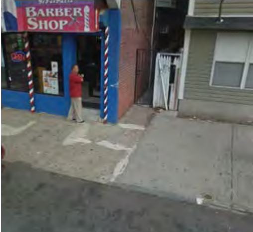
Figure 73. Existing sidewalks cracked and patched with very little curb.
