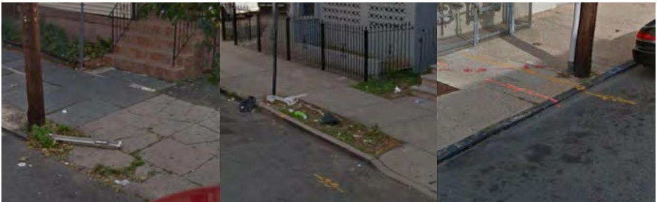
Figure 69. Existing sidewalks: Cracked driveway with bluestone slabs in background (L); 2-foot planting strip filled with litter (C); 3-inch granite curb height (R)
