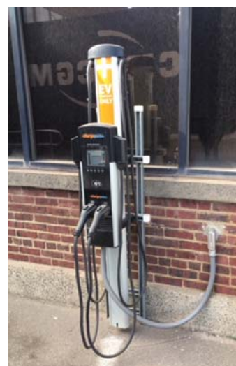
Workplace charging at Bayshore Recycling Photo courtesy of Bayshore Recycling
